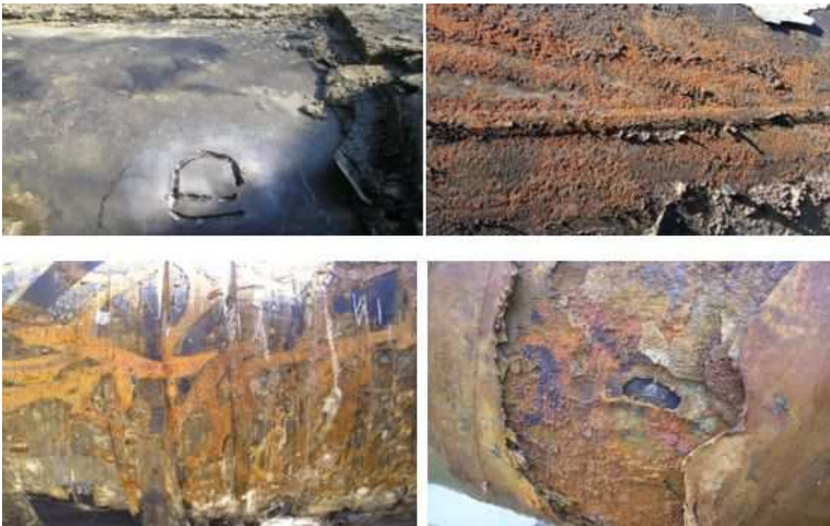
Figure 10 – Pipe body defects
